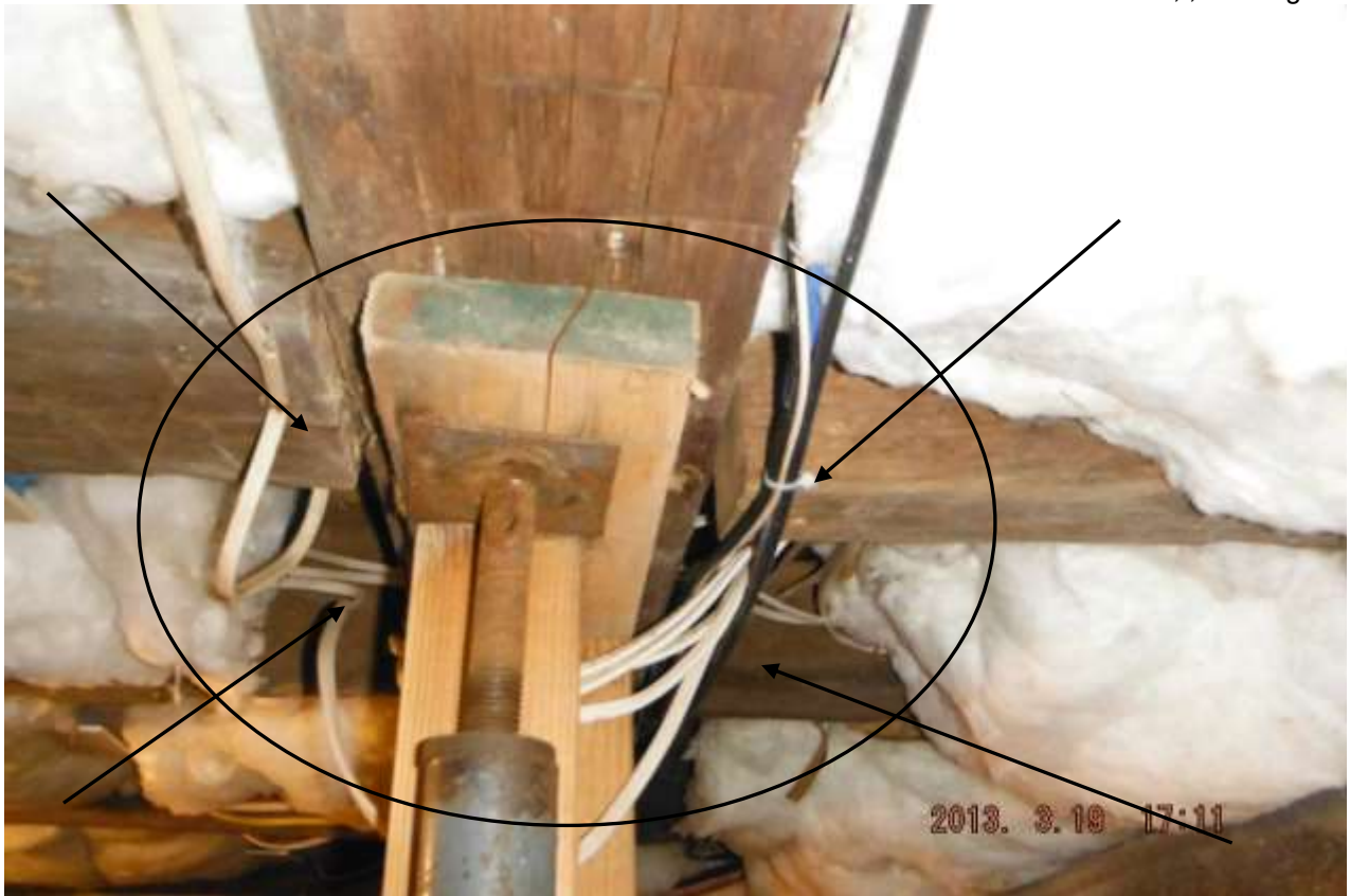
Figure 47 Improperly repaired structure in basement; handyman or improper.
