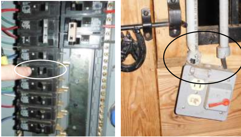
Figure 35 Breaker buzzed and tripped. Numerous extension cords and devices plugged into outlets in stalls; overloaded/fire safety concern. There was a damaged outlet mounted on outside of a stall approximately half way down center.
