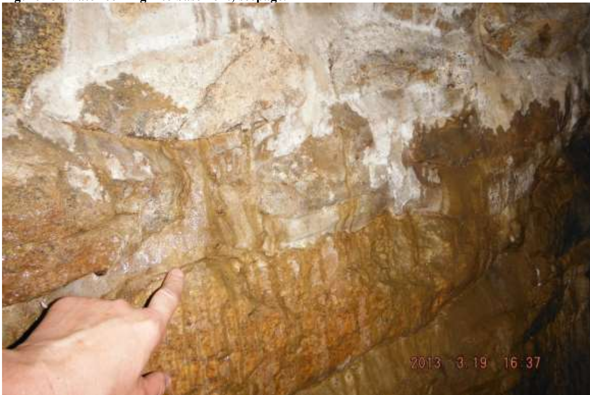
Figure 26 Water coming into basement; seepage.
