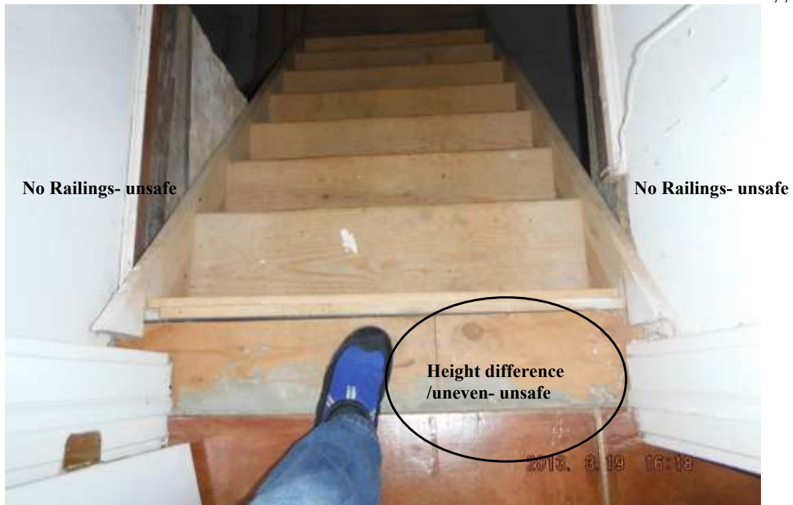
Figure 39 Have a contractor or carpenter repair the uneven heights between the kitchen floor and the wood just inside the basement at top of steps. Add railings for safety, and on basement landing to right; safety hazard. Have stringers trimmed at bottom; trip hazard.
