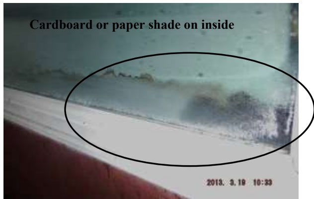
Figure 11 Example of vapor seal breaks on guesthouse windows; older thermo pane type. Have a window installer evaluate all windows and make repairs/replacement where needed.
