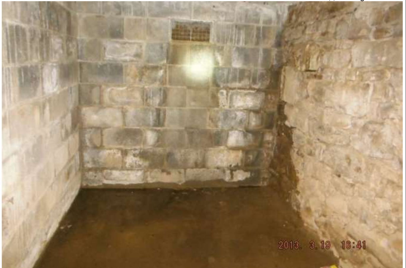
Figure 24 Water coming into basement; seepage.
