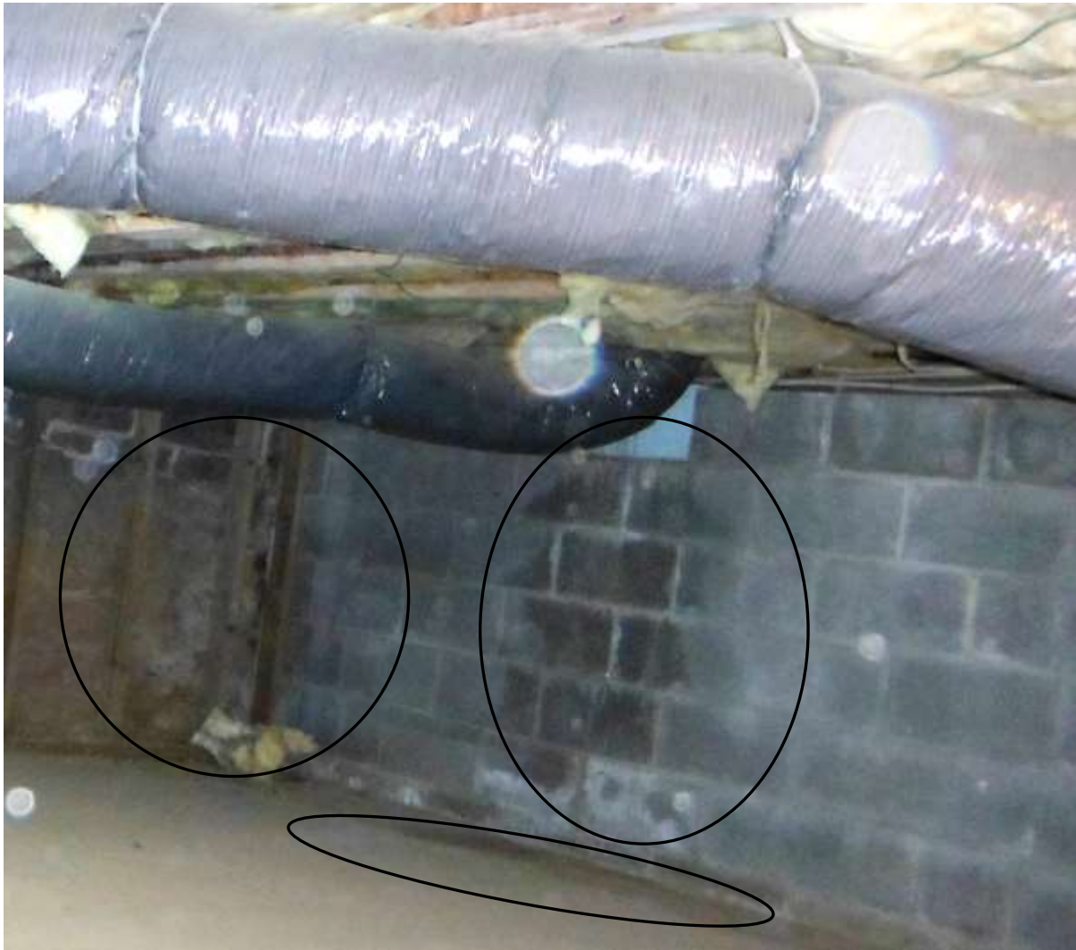
Figure 23 Seepage in crawl space and vents were closed with foam. Moisture needs to be removed; correct grading & drainage, gutters and installer dehumidifier.
