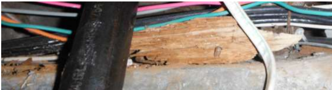
Figure 16 Termites damage sills, joists, sub-flooring in basement. Have structural carpenter determine the extent of damage.
