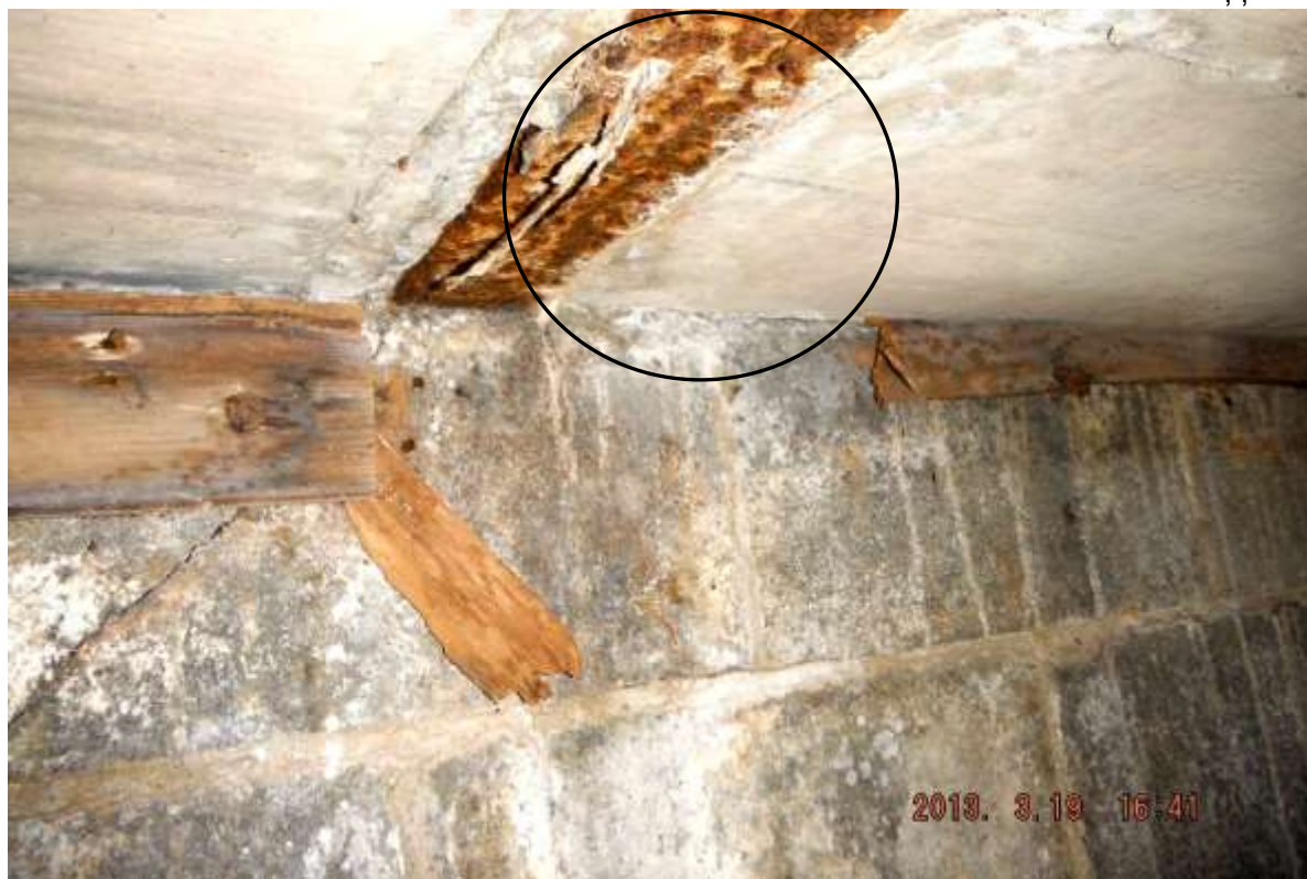
Figure 41 Corroded metal floor supports under front steps in well storage room. There was termite damage on wood in front room.
