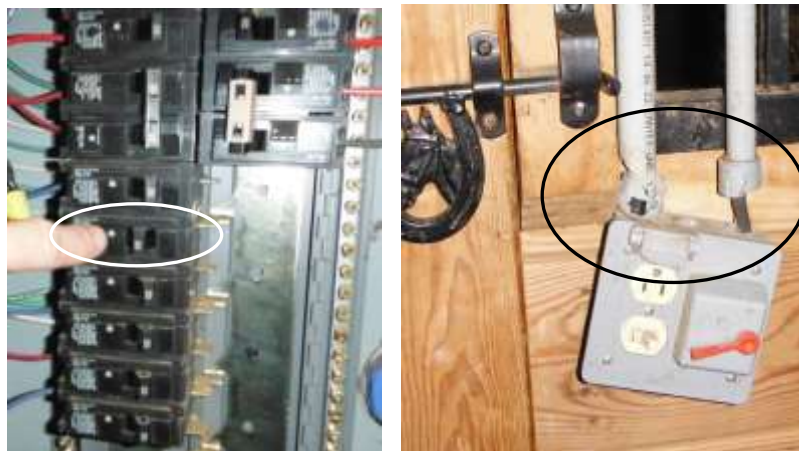
Figure 9 Breaker buzzed and tripped. Numerous extension cords and devices plugged into outlets in stalls; overloaded/fire safety concern. There was a damaged outlet mounted on outside of a stall approximately half way down center.
