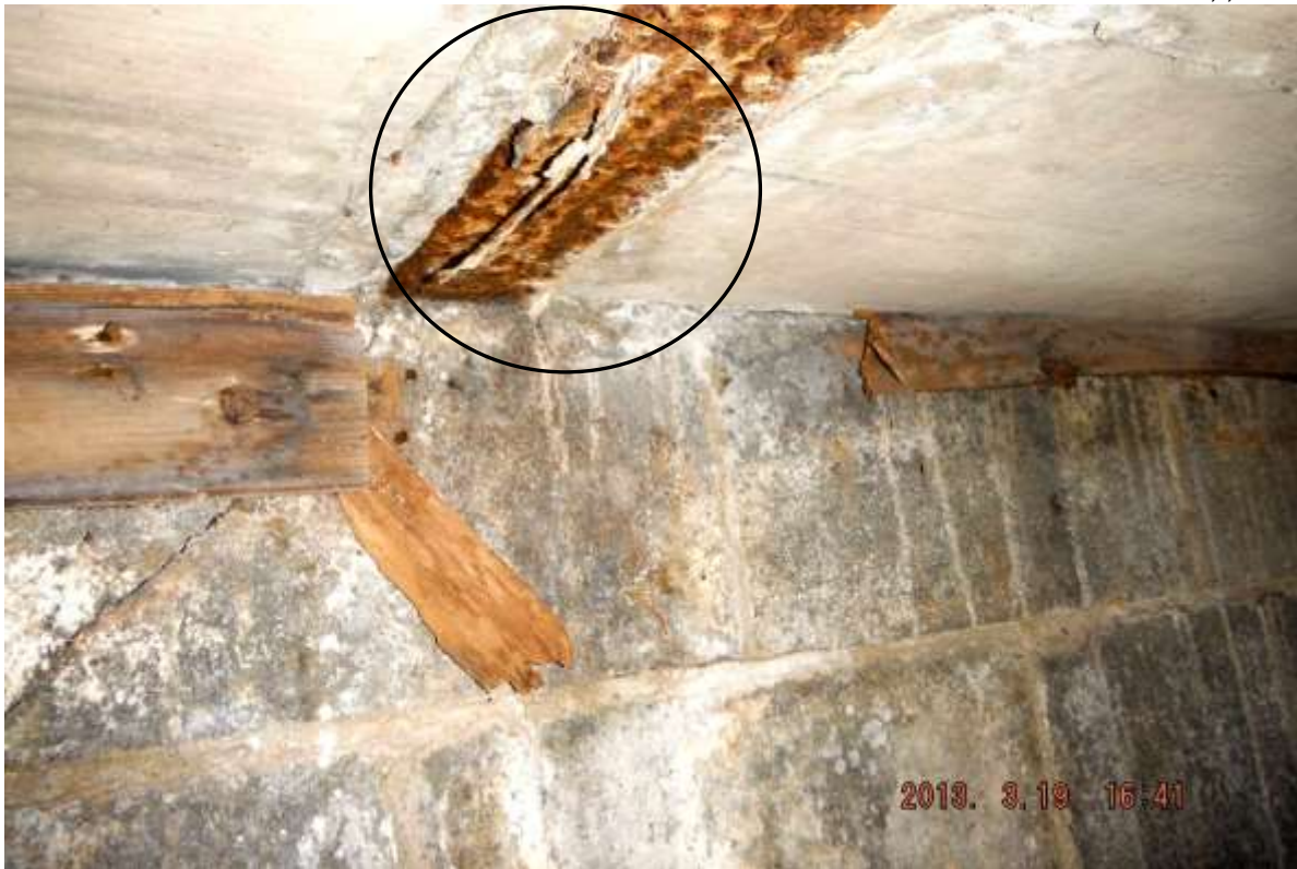
Figure 15 Corroded metal floor supports under front steps in well storage room. There was termite damage on wood in front room.
