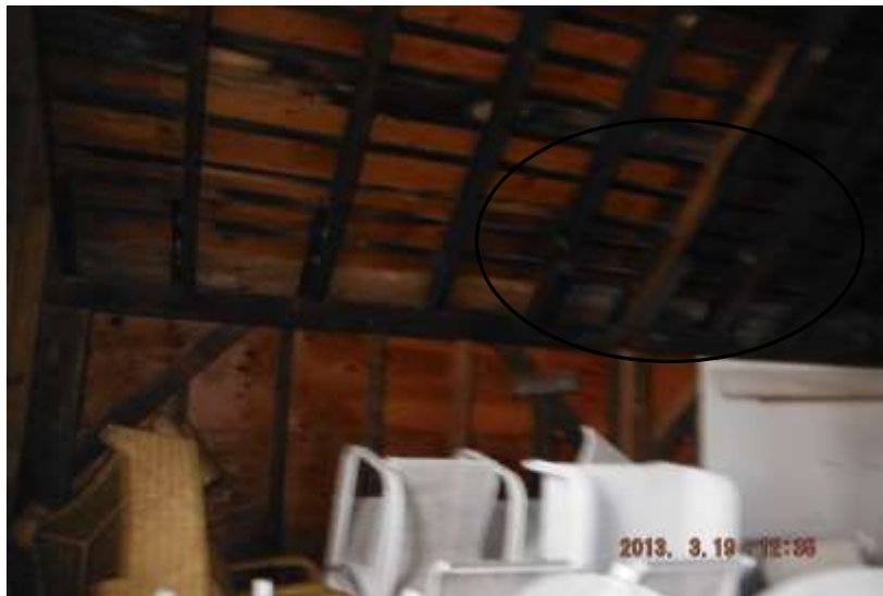
Figure 30 Garage had old asphalt roof. There were water stains visible inside from second floor; leaking.
