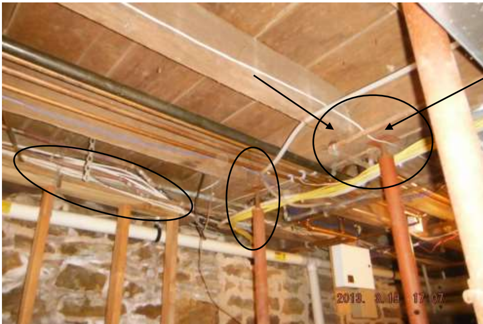
Figure 48 Have structural engineer or qualified building contractor evaluate repairs and structure in home.
