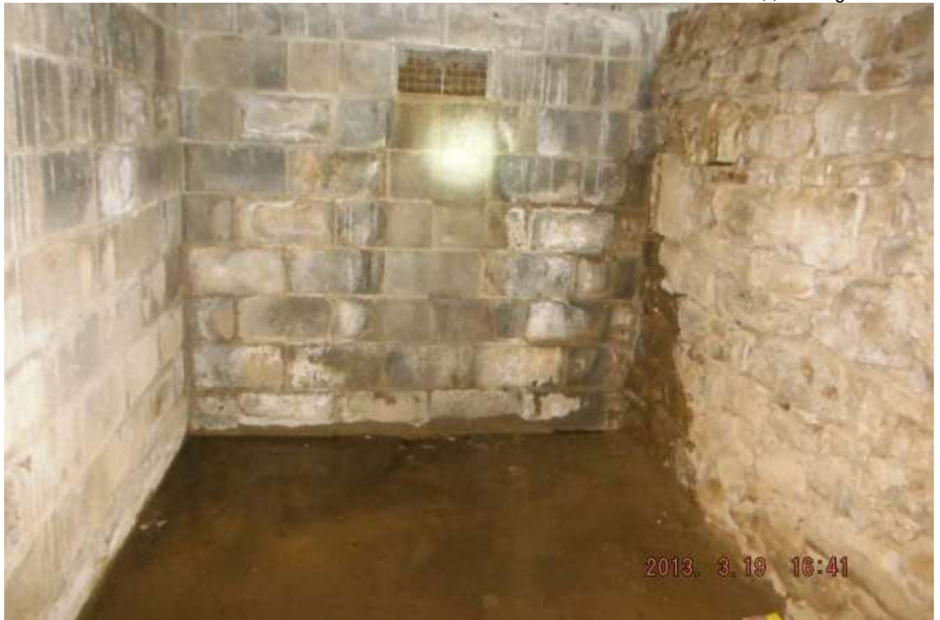
Figure 50 Water coming into basement; seepage.
