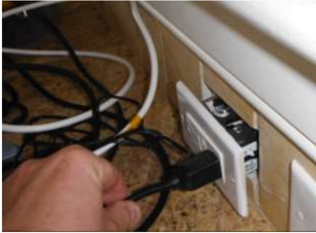
Figure 36 Have outlet repaired by electrician; shock hazard.
