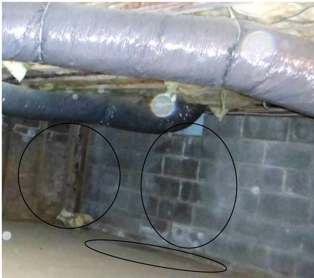
Figure 49 Seepage in crawl space and vents were closed with foam. Moisture needs to be removed; correct grading & drainage, gutters and install dehumidifier.
