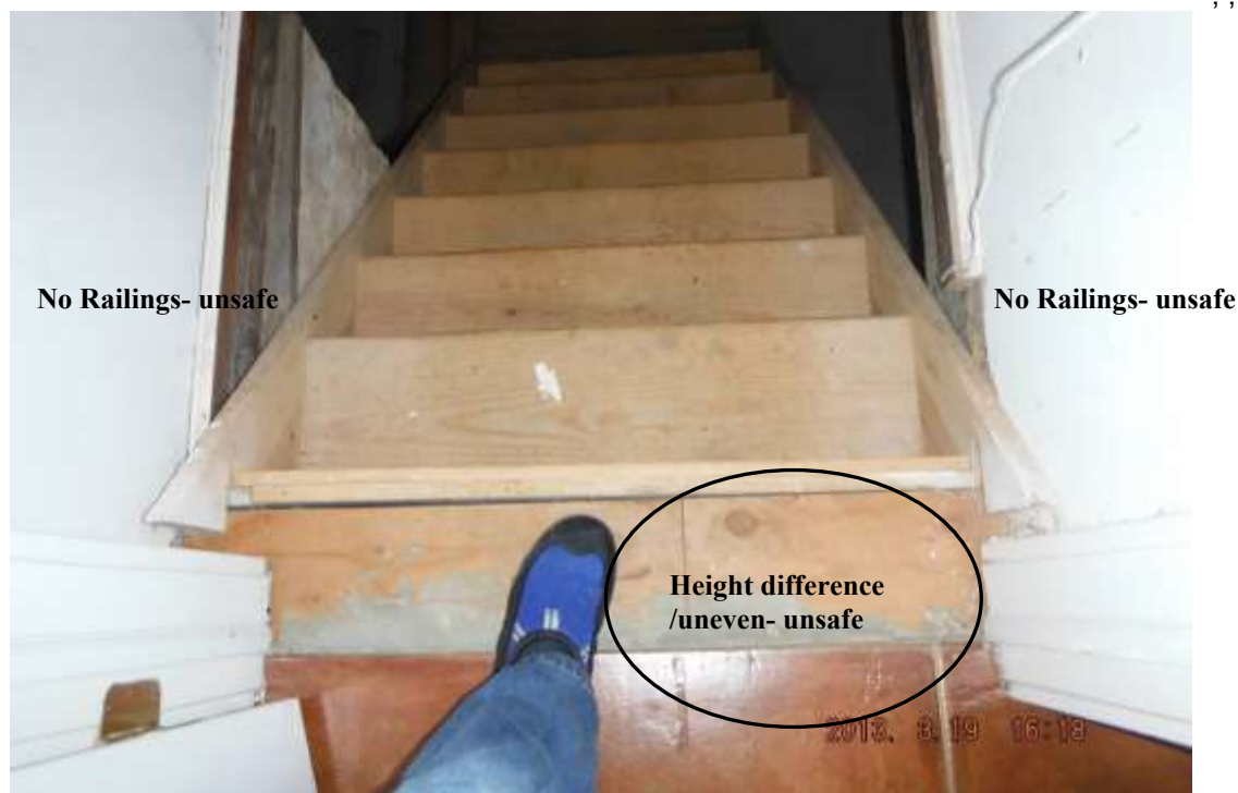
Figure 13 Have a contractor or carpenter repair the uneven heights between the kitchen floor and the wood just inside the basement at top of steps. Add railings for safety, and on basement landing to right; safety hazard. Have stringers trimmed at bottom; trip hazard.
