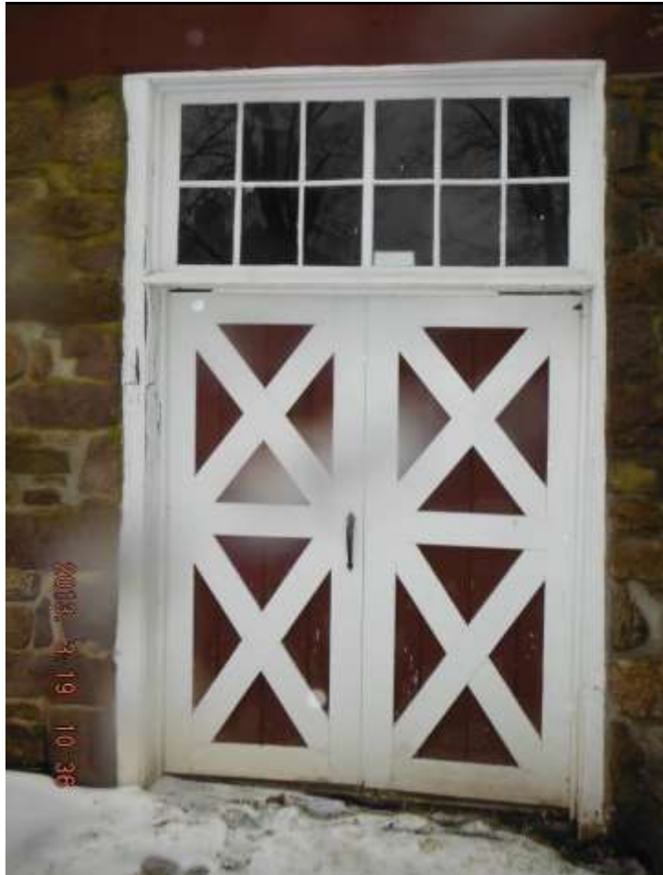
Figure 33 Guesthouse exterior water damage on side door and window units. Have window & door installer evaluate for replacement/repairs and flashings. Gutters need to be addressed on all buildings.
