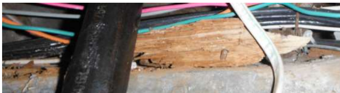
Figure 42 Termites damage sills, joists, sub-flooring in basement. Have structural carpenter determine the extent of damage.
