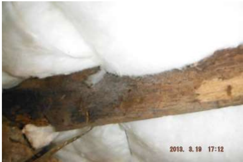
Figure 18 Example of powder post beetle damage. Have a structural carpenter determine extent of all wood destroying insect damage before closing.
