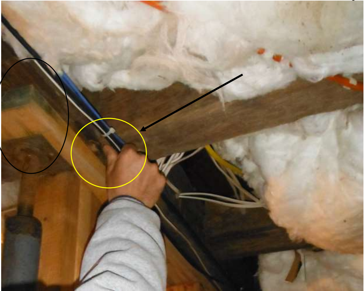
Figure 20 Handyman repairs; have structural engineer evaluate repairs and structure and advise on all needed structural repairs.
