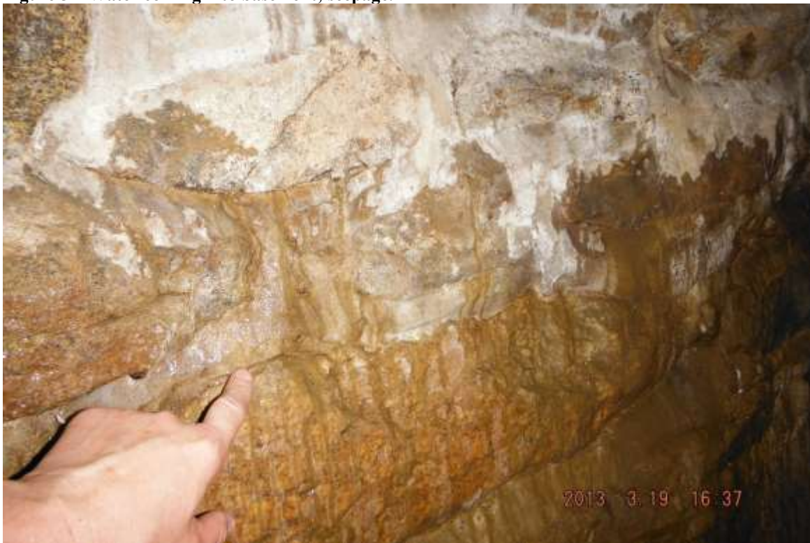
Figure 52 Water coming into basement; seepage.
