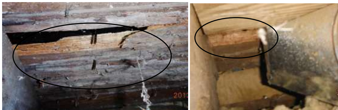
Figure 43 Termites damage sills, joists, sub-flooring in basement. Have structural carpenter determine the extent of damage.
