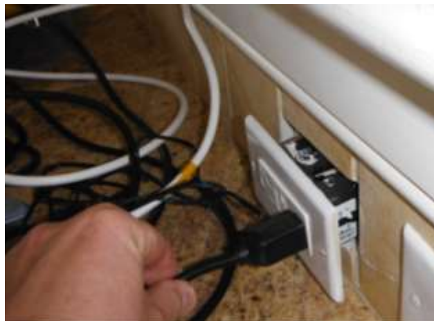
Figure 10 Have outlet repaired by electrician; shock hazard.
