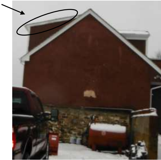
Figure 29 Low sloped roof appeared to be tab asphalt (view on edge of snow covered roof). Asphalt shingles on pitches lower than 4/12 are prone to leaks.
