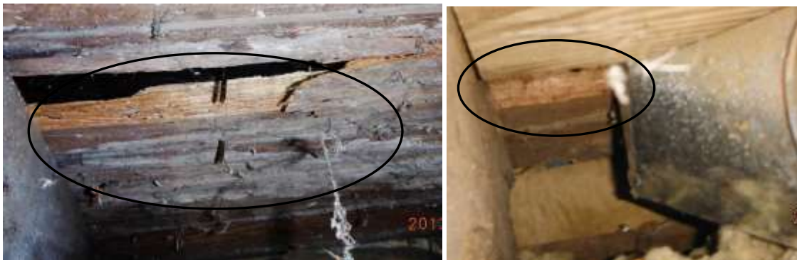
Figure 17 Termites damage sills, joists, sub-flooring in basement. Have structural carpenter determine the extent of damage.
