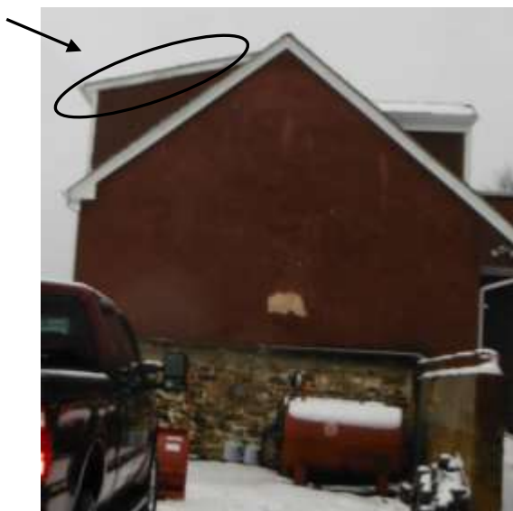
Figure 3 Low sloped roof appeared to be tab asphalt (view on edge of snow covered roof). Asphalt shingles on pitches lower than 4/12 are prone to leaks.
