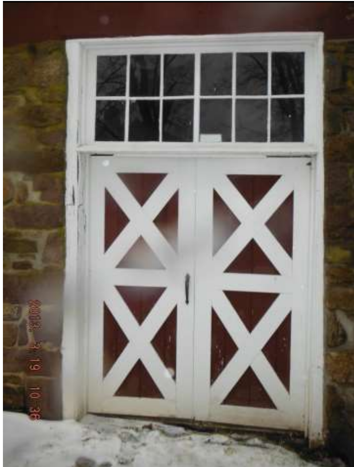
Figure 7 Guesthouse exterior water damage on side door and window units. Have window & door installer evaluate for replacement/repairs and flashings. Gutters need to be addressed on all buildings.
