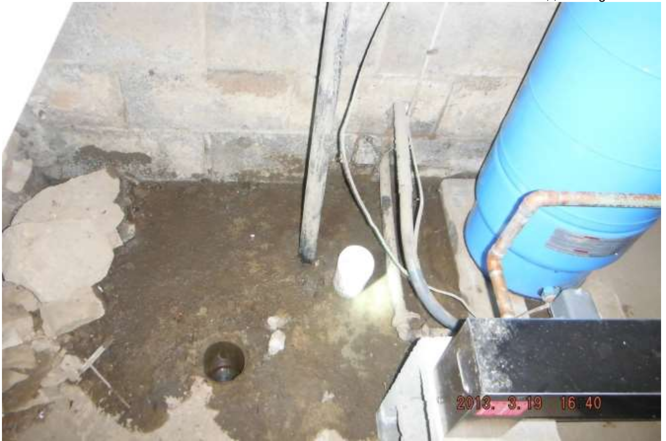
Figure 25 Water coming into basement; seepage.
