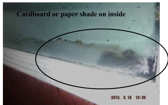
Figure 37 Example of vapor seal breaks on guesthouse windows; older thermo pane type. Have a window installer evaluate all windows and make repairs/replacement where needed.
