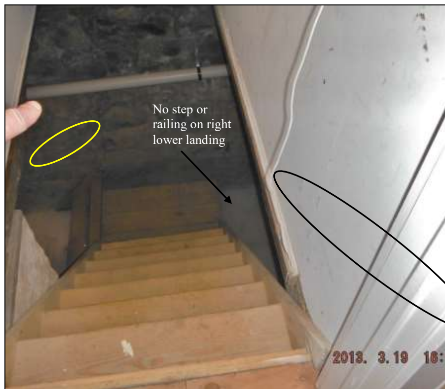
Figure 14 Lower landing unsafe; no railing or step to right side. Recommend railing on all steps.
