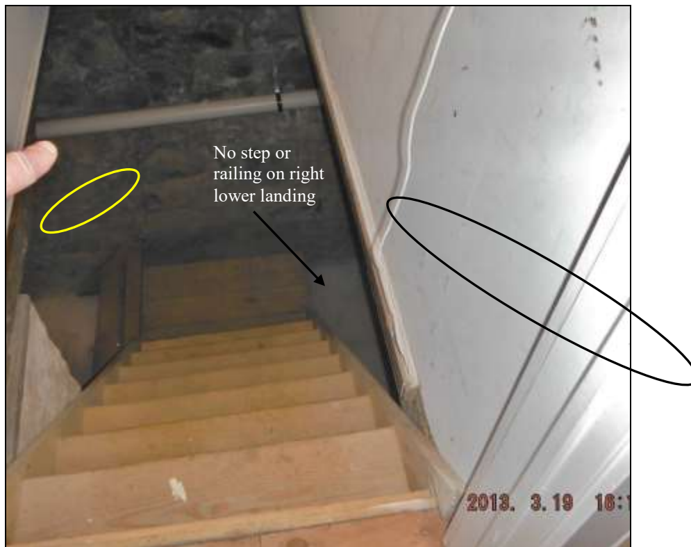
Figure 40 Lower landing unsafe; no railing or step to right side. Recommend railing on all steps.
