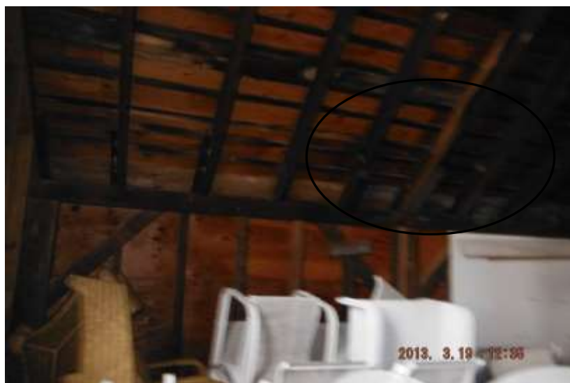
Figure 4 Garage had old asphalt roof. There were water stains visible inside from second floor; leaking.
