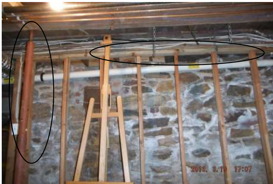
Figure 45 Have all structural repairs evaluated by a structural engineer or qualified building contractor before closing. There were structural concerns and handyman repairs.
